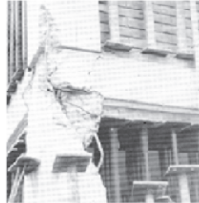
Foto tomada de la Figura 149, Failure of Column and Beam Connection, Column A1. "The Venezuela Earthquake", July 29, 1967 by Robert D. Hanson (15)
